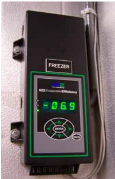
The controller, installed outside of the refrigerated space, displays the temperature in tenths of a degree, and is visible without entering the freezer.
