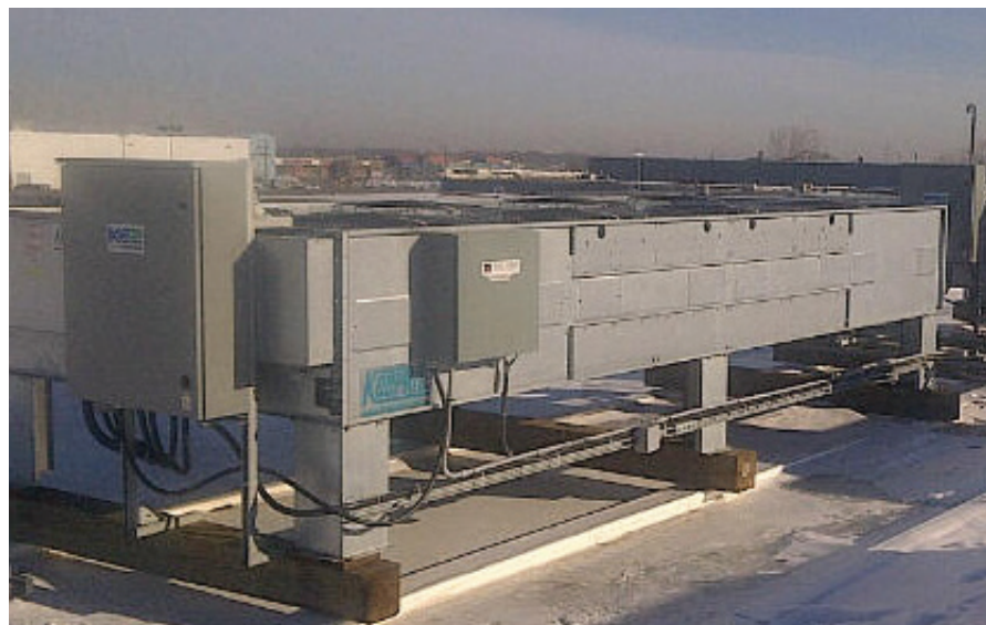
A 8 fan KE2 Fan Control installation at Costco in Pointe Claire Quebec. The unit has been in operation with the KE2 Fan Control in place since 2012 and has provided an estimated 57% energy savings.
