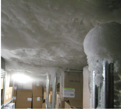
Figure 3 - Before - Severe ice problem
